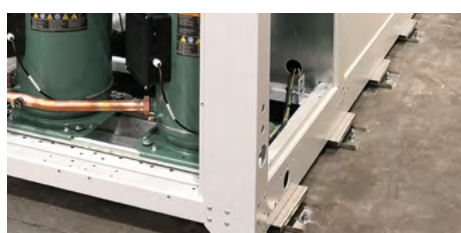
Chiller air conditioning system
