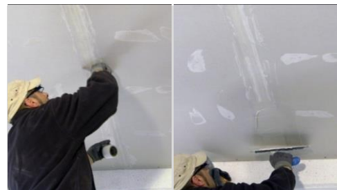
Apply the plastic mesh tape in the gypsum boards jointing lines and grouting
