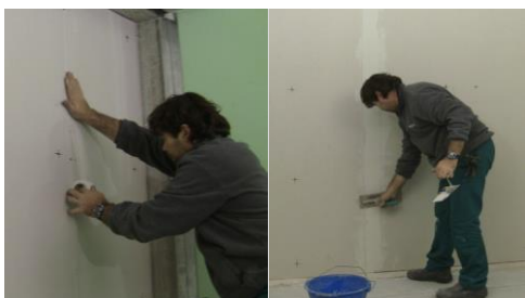
Apply the plastic mesh tape in the gypsum boards jointing lines. Grouting
